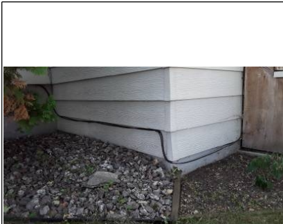
Soil to close to siding to prevent damage to siding/framing recommend a clearance of 6-8" to grading be maintained.
