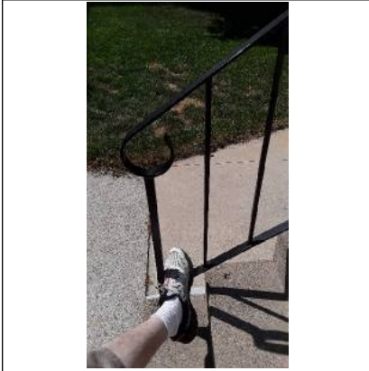
For enhanced safety recommend 4" max spacing between balusters.
